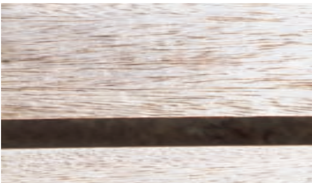
Iroko finished in Cuprinol exterior wood stain after 18-24 months
